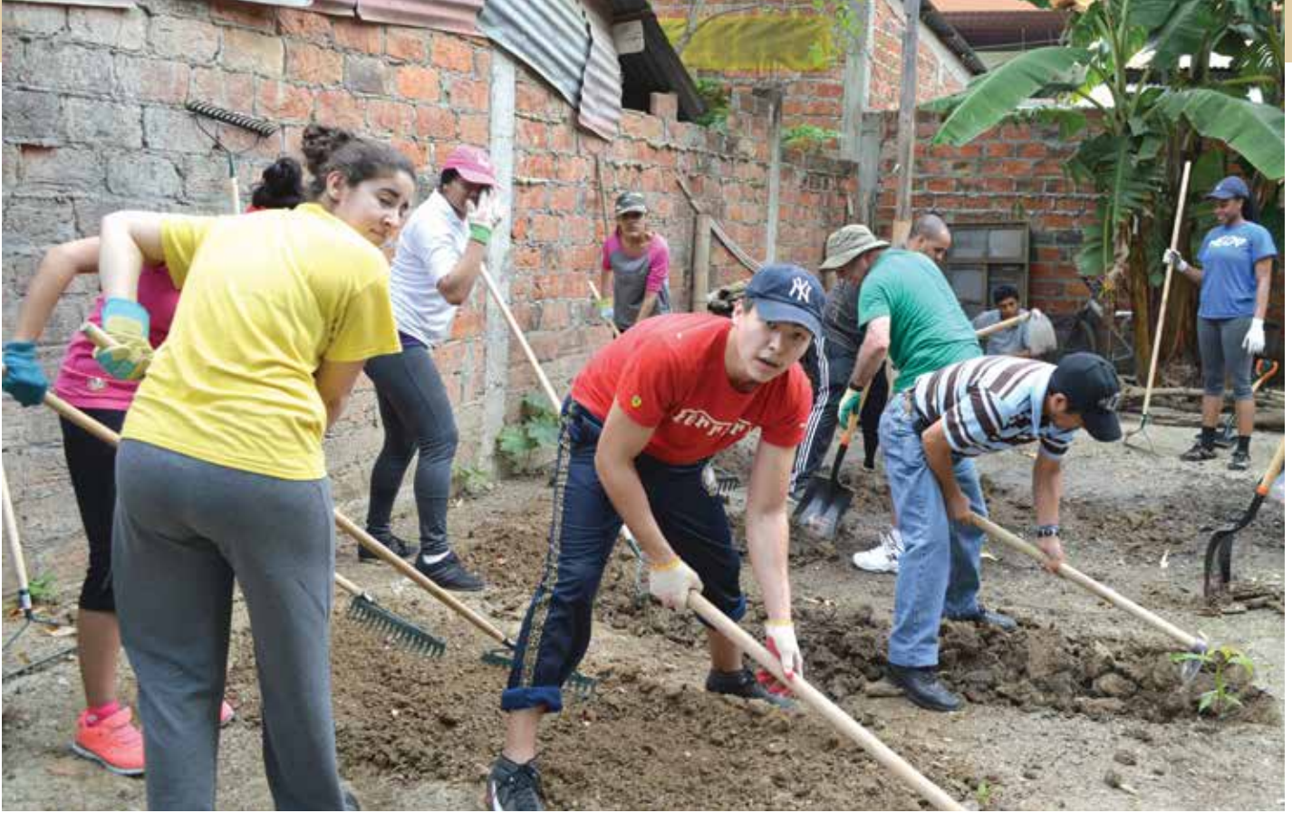
■ As part of 2014 Alternative Spring Break in Ecuador, NYIT students and staff join staff members from ACJ Ecuador to build an organic garden for a family whose home had been damaged in a recent flood.
